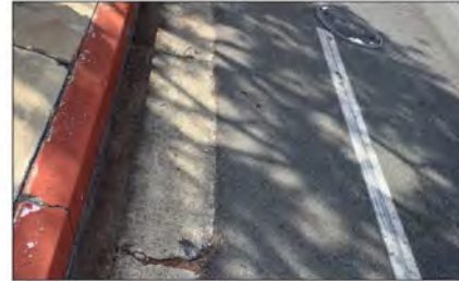
7 Bike lane narrow and uneven, especially for a high speed roadway
